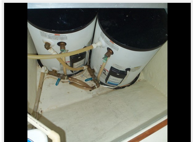
Water Heaters Below VIP
