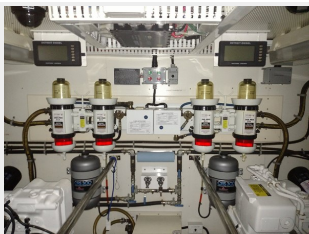
Engine Room Forward
