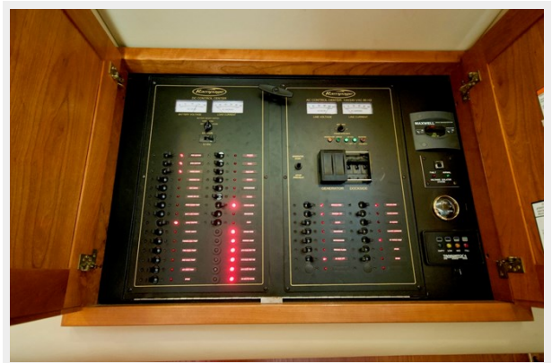
Main Distribution Panel
