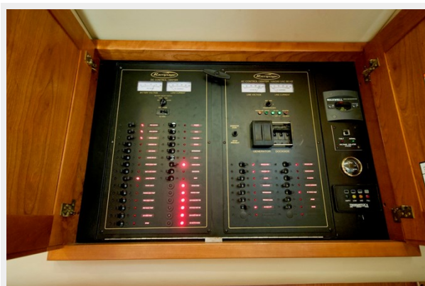
Main Distribution Panel
