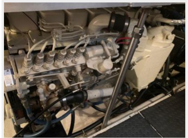
57 Summer Place 2000 Carver 406 engine room 5
