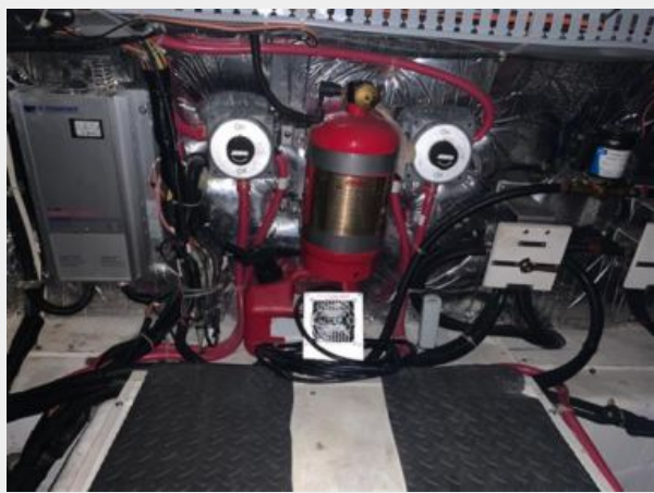
55 Summer Place 2000 Carver 406 Engine Room 4
