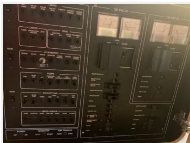
62 Summer Place 2000 Carver 406 electrical panel 1
