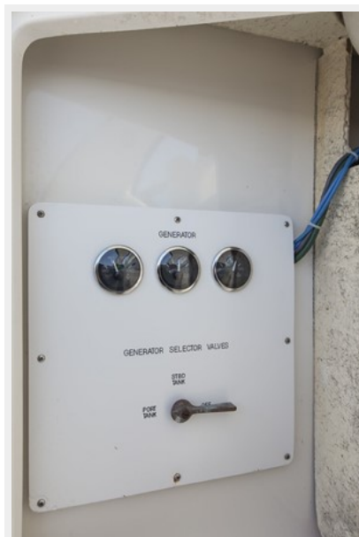
Generator selector valves
