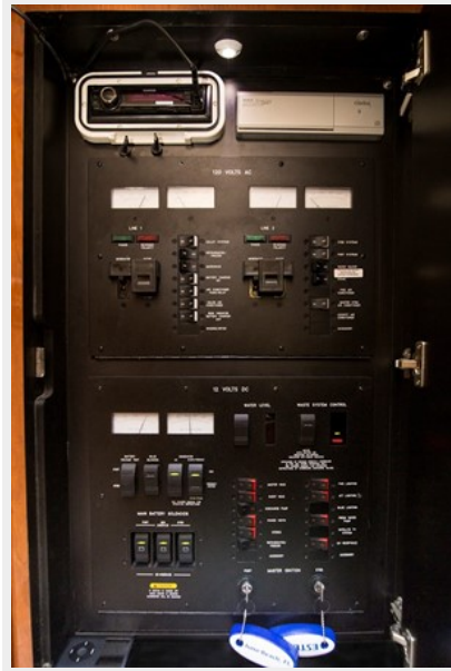
Control panel Galley
