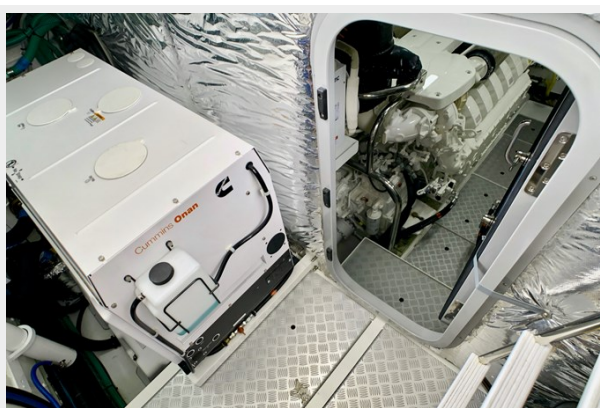
2019 Princess 70 Flybridge Engine Room
