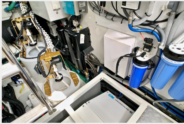
2019 Princess 70 Flybridge Engine Room
