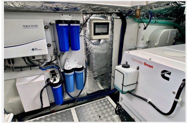
2019 Princess 70 Flybridge Engine Room
