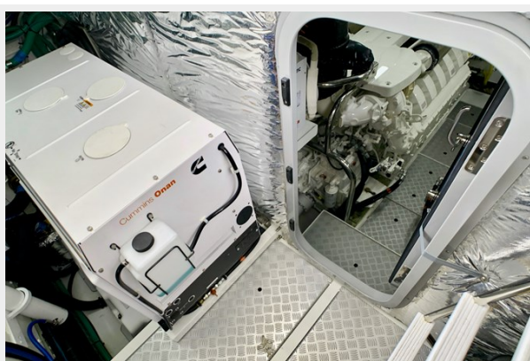
2019 Princess 70 Flybridge Engine Room
