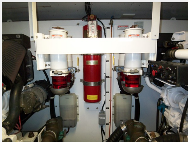
Engine Room Forward
