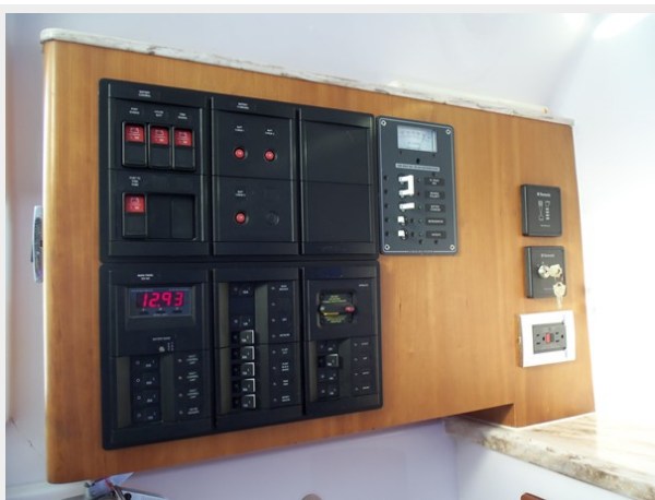
Console Electrical Panel
