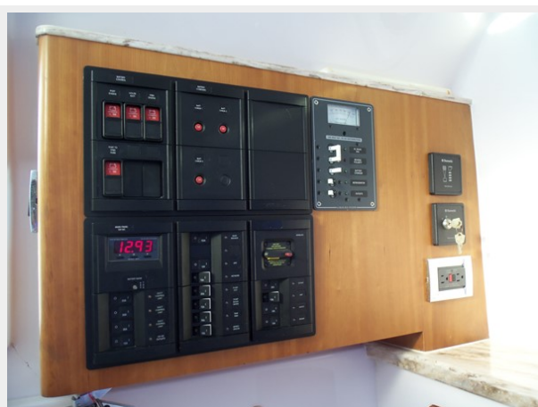
Console Electrical Panel
