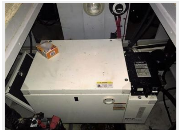
41.1 The Blessing 2000 Silverton 352 Generator
