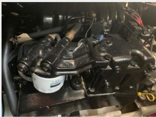
37 The Blessing 2000 Silverton 352 Engine Room 3
