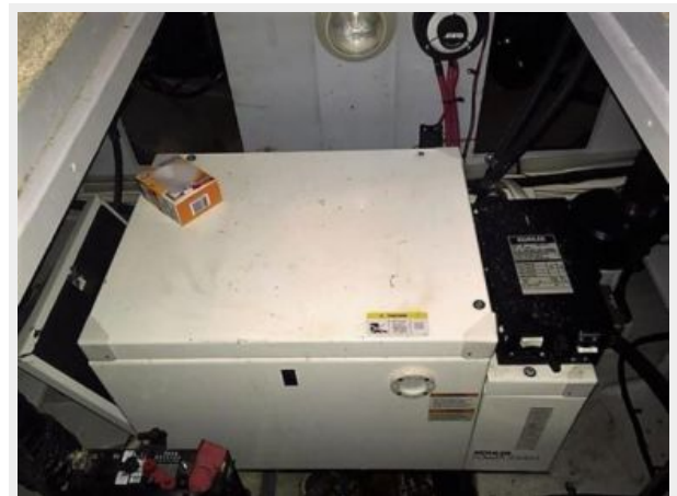
41.1 The Blessing 2000 Silverton 352 Generator
