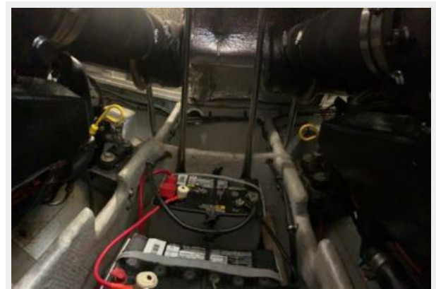
36 The Blessing 2000 Silverton 352 Engine Room 2
