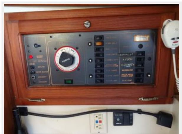
011 Electrical distribution panel
