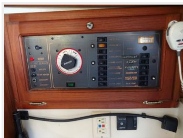
011 Electrical distribution panel
