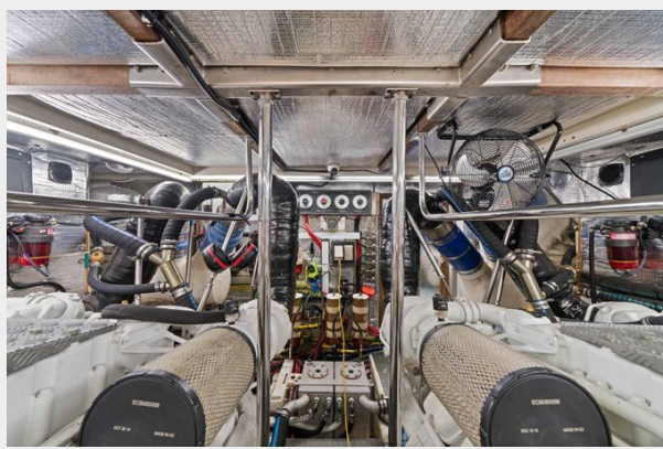
Engine Room Looking Aft
