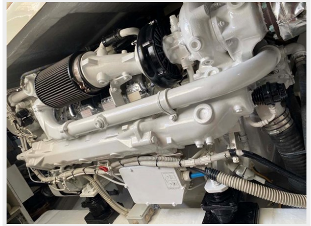
Engine Room Full Detail 2022
