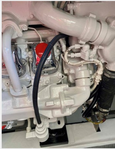
Engine Room Full Detail 2022
