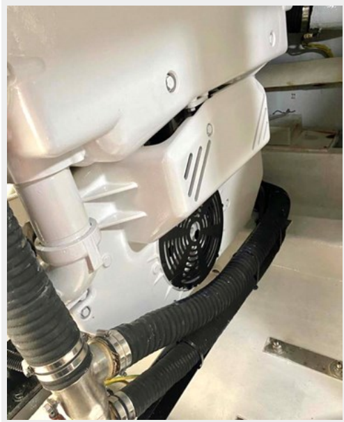
Engine Room Full Detail 2022
