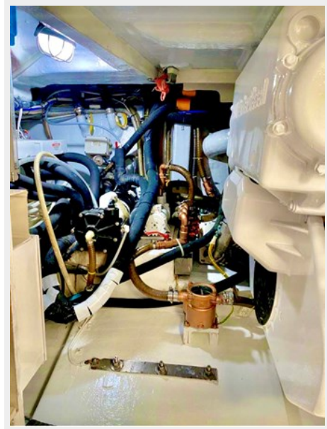
Engine Room Full Detail 2022
