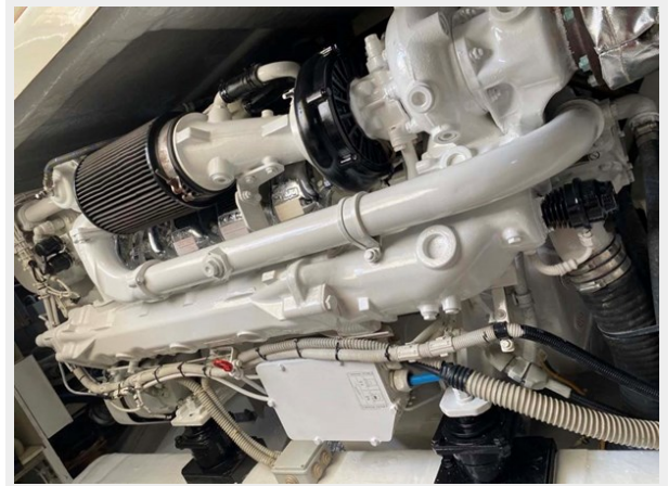
Engine Room Full Detail 2022
