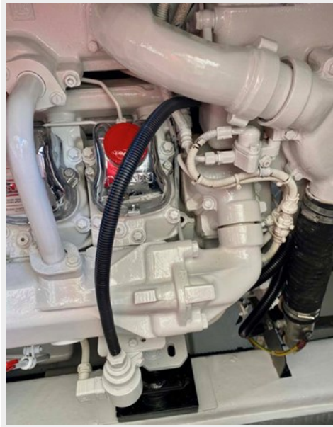
Engine Room Full Detail 2022
