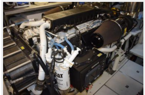
Starboard main engine
