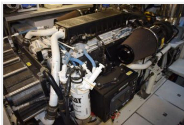
Starboard main engine
