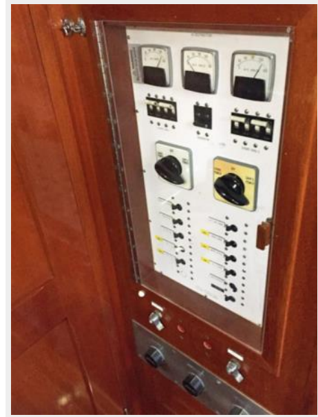
AC Electrical Panel
