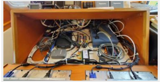
34 screens down wiring close
