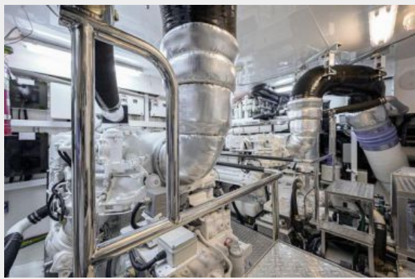
Wiggle Room_Engine Room7
