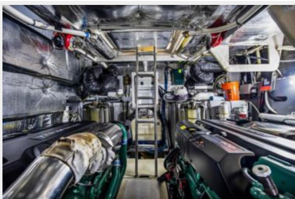
Infinito Engine Room 2
