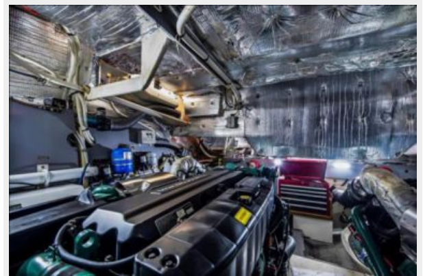
Infinito Engine Room 1
