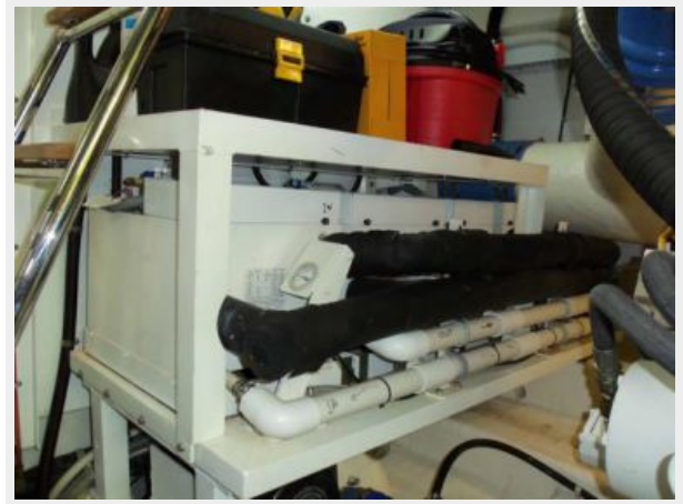
Chilled Water AC New 2019
