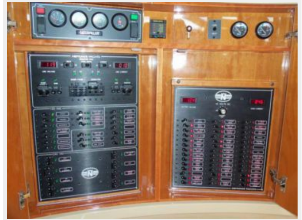
Main Electrical Panel
