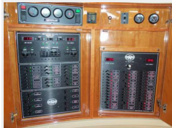
Main Electrical Panel
