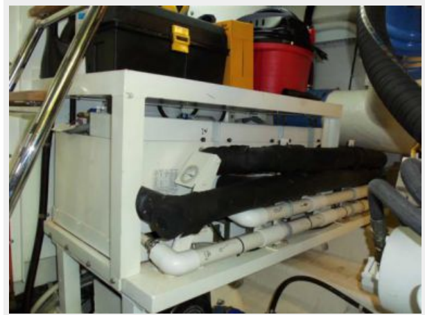
Chilled Water AC New 2019
