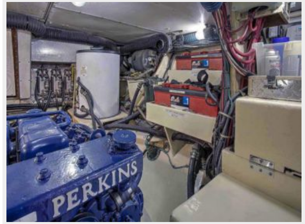
Engine Room, Fwd.
