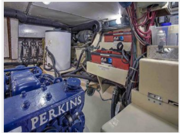
Engine Room, Fwd.
