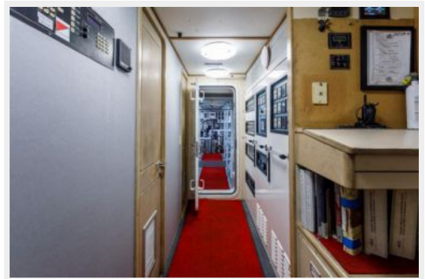
Engine Room Hallway
