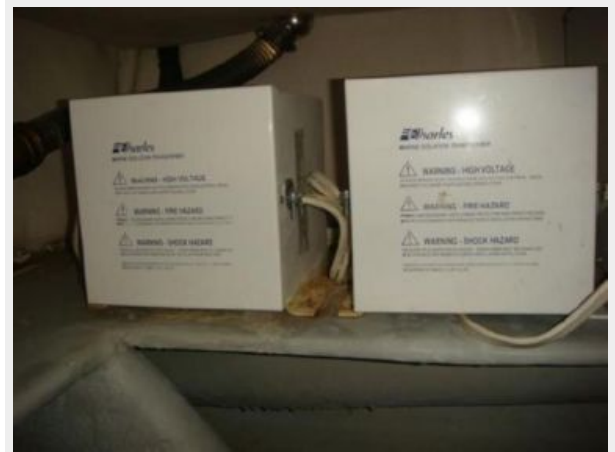
312 Charles Isolation Transformers
