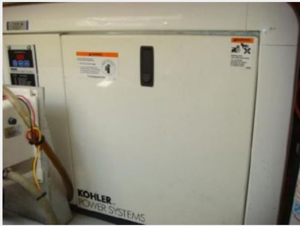
309 Generator Sound Shield
