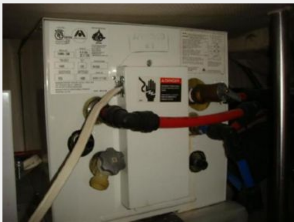
311 Hot Water Htr
