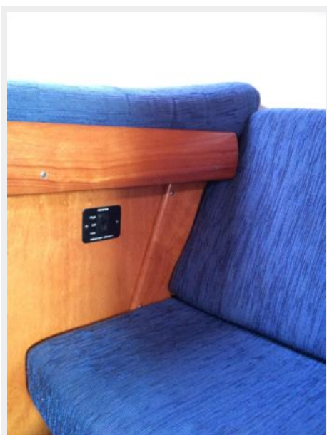
Diesel heat control
