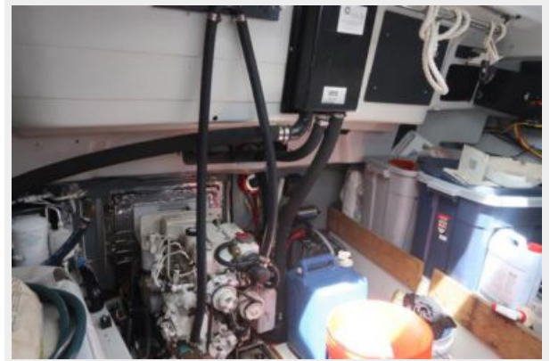
42 Genset in Lazerette
