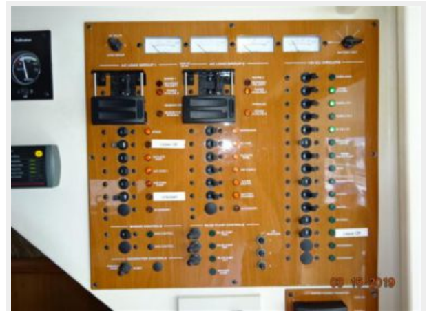
37ELEC Electrical Panel
