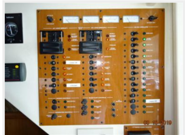
37ELEC Electrical Panel
