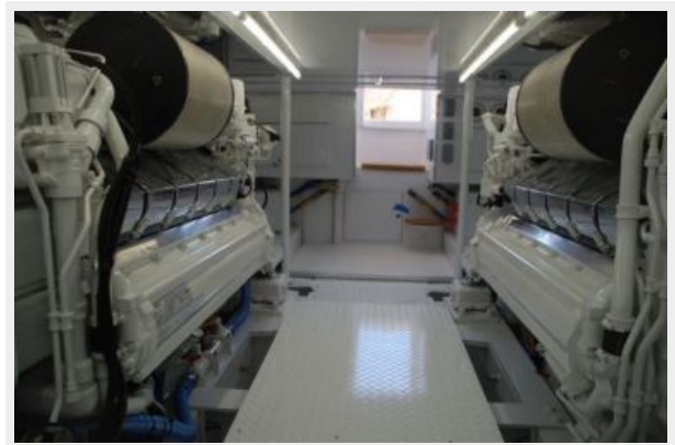
Engine room aft
