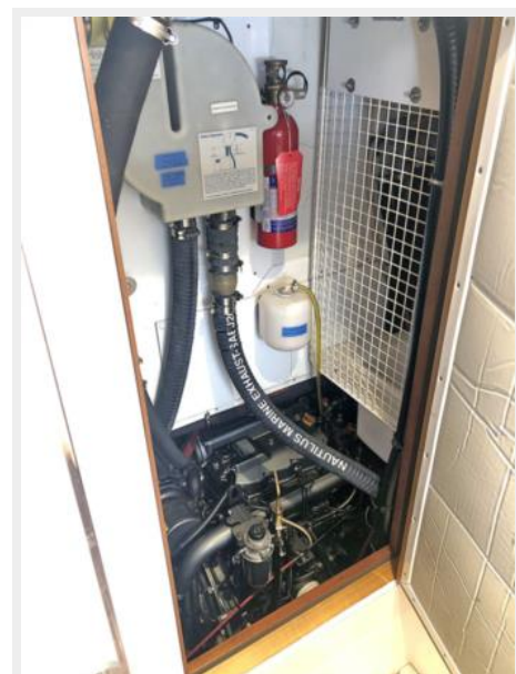
Engine Room, Fwd.
