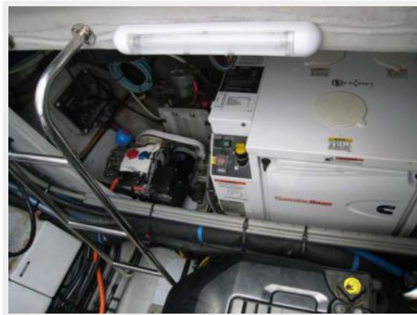
Engine Room - Generator
