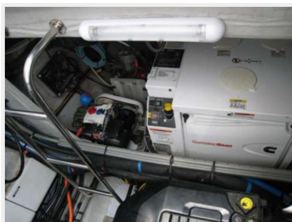
Engine Room - Generator
