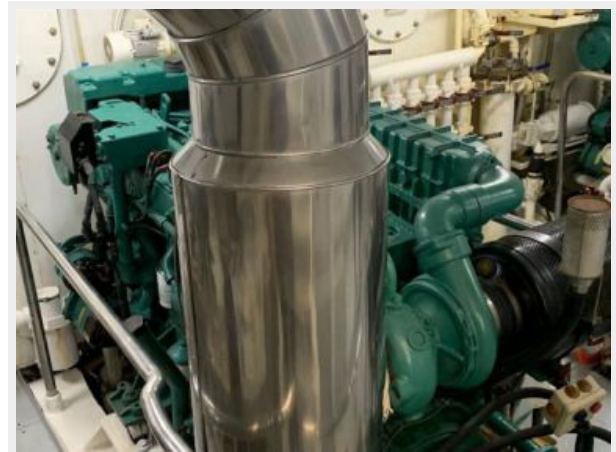
20.Victoria A_engine room5
