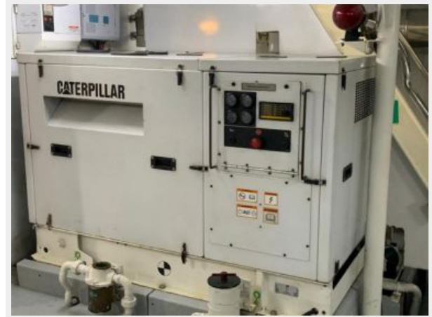
20.Victoria A_engine room3
