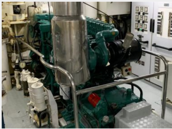
20.Victoria A_engine room2
