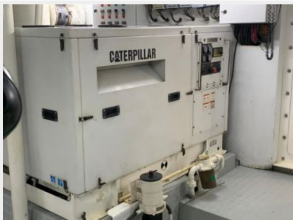
20.Victoria A_engine room4
