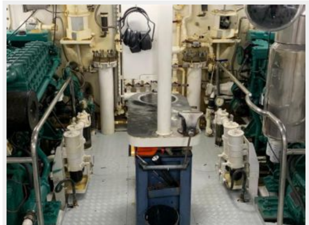
20.Victoria A_engine room1
