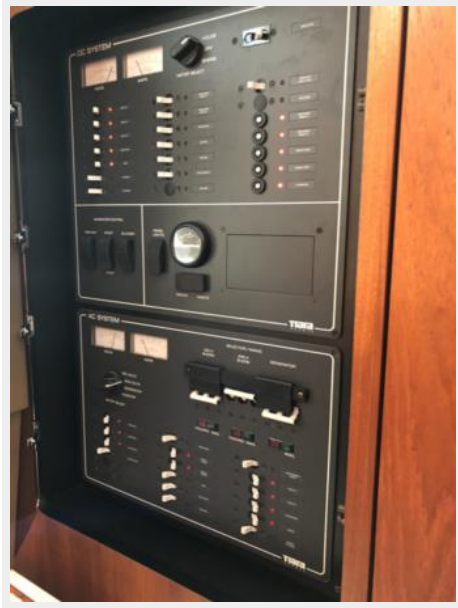
40 Tiara Breaker Panel
