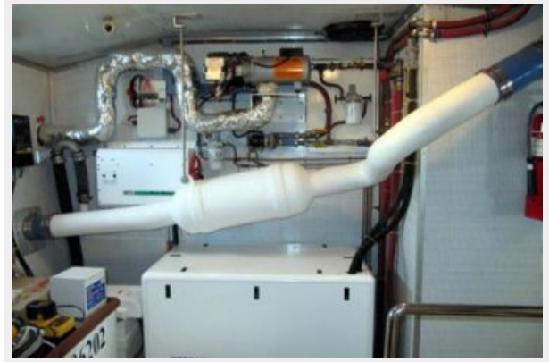
GENERATOR WITH HUSH COVER
