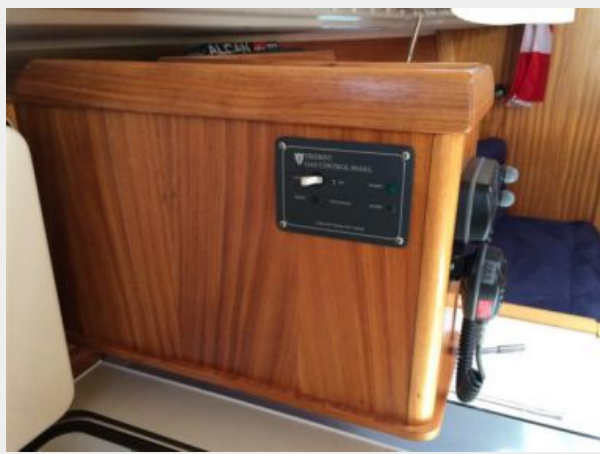
Propane Remote Control Panel
