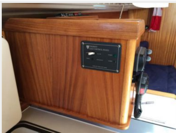
Propane Remote Control Panel
