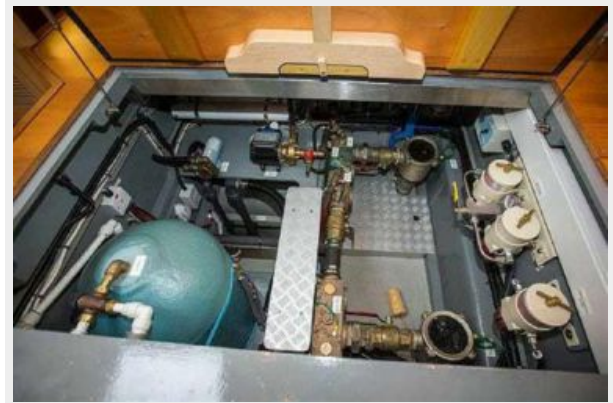
Easy Access to Plumbing
