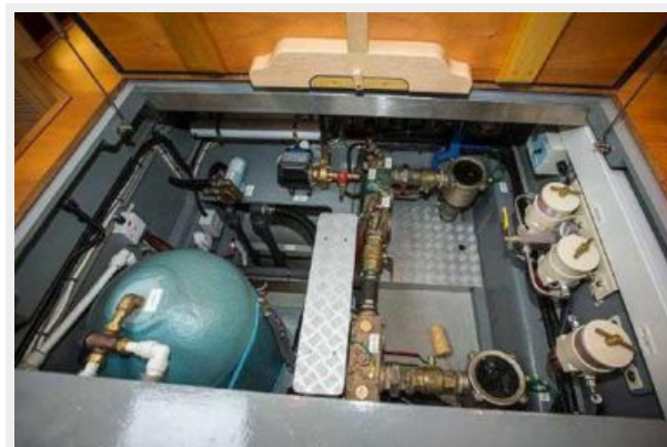
Easy Access to Plumbing
