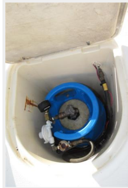
Propane locker (1 of 2)
