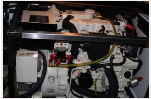
Generator with cover off
