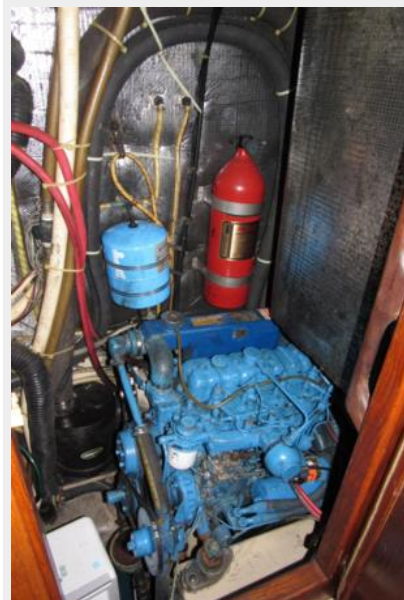
Engine room from walkthrough
