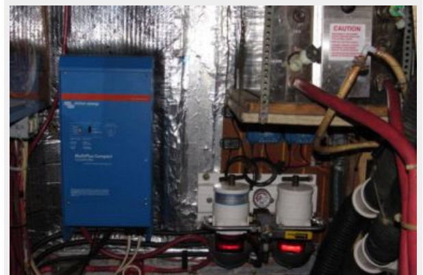
Inverter & fuel filters
