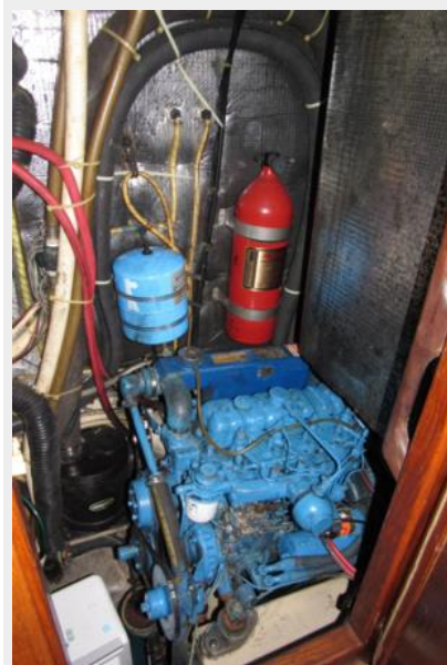
Engine room from walkthrough
