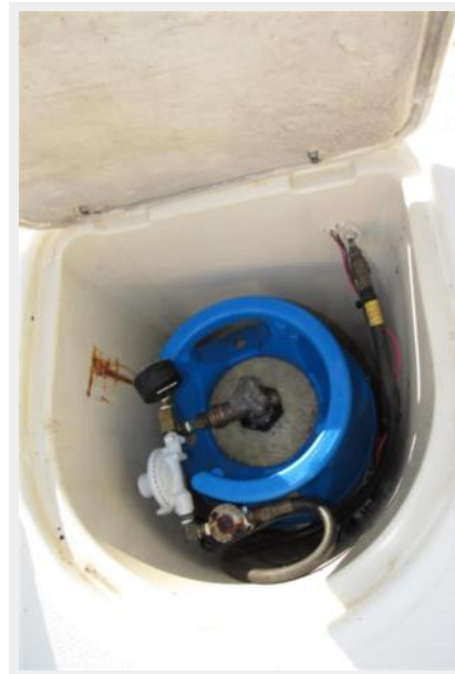
Propane locker (1 of 2)
