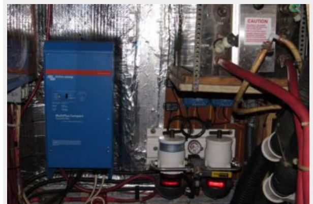
Inverter & fuel filters
