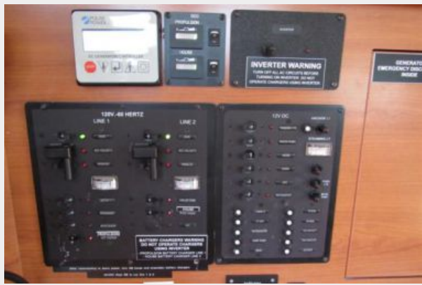
Electrical panel, regulator etc
