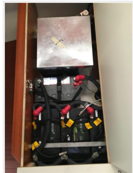
Batteries and water heater
