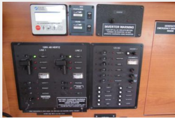
Electrical panel, regulator etc
