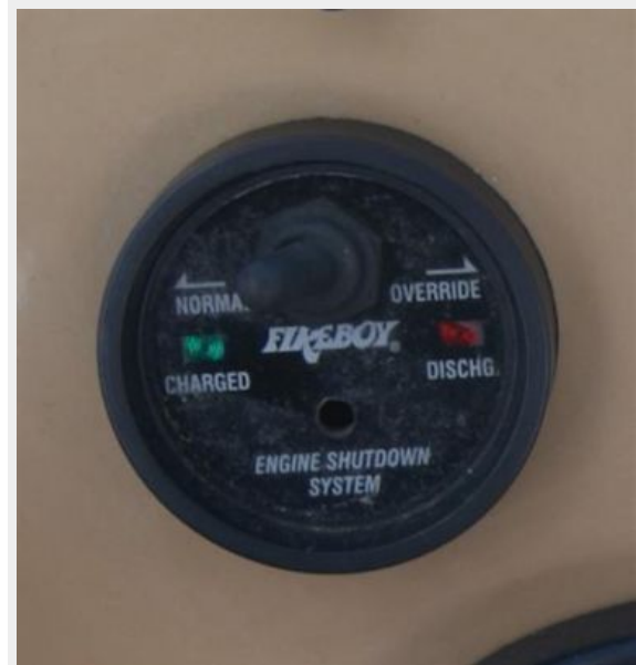
311 FireBoy Engine Shutdown
