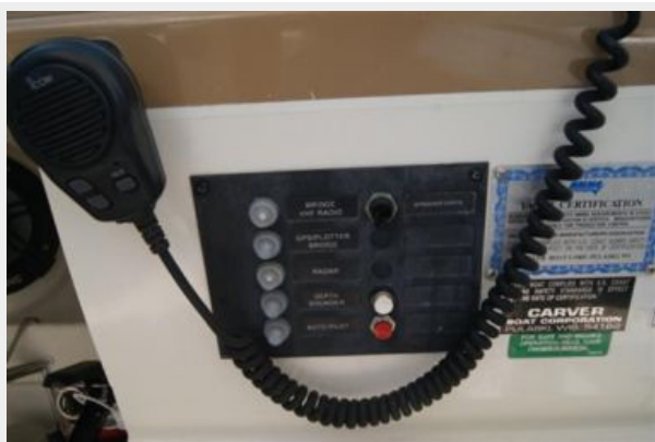
318 Bridge 12v Breakers
